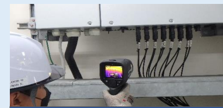
Maintenance (equipment inspection)
