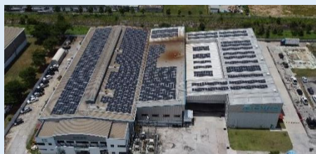
DOWA THERMOTECH (THAILAND) 498.96 kW
