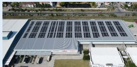
FUJITSU GENERAL (THAILAND) Factory2 998.46 kW
